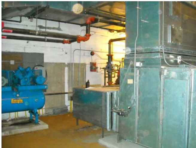
HVAC-1 – Building H Central Station Air Handling Unit
