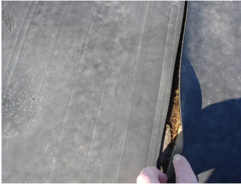
Figure 29. Split at EPDM roofing membrane over library.
