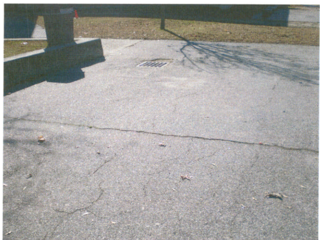
Concrete cracking in courtyard
