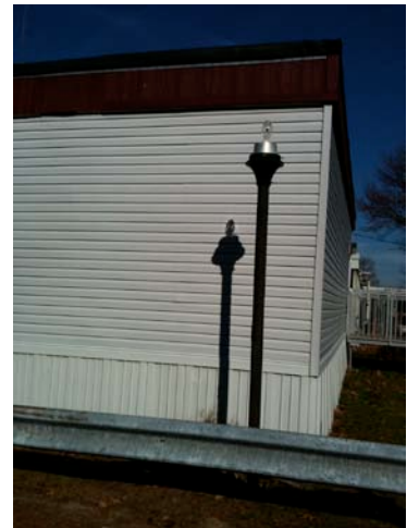
Low Level Pole Lighting
