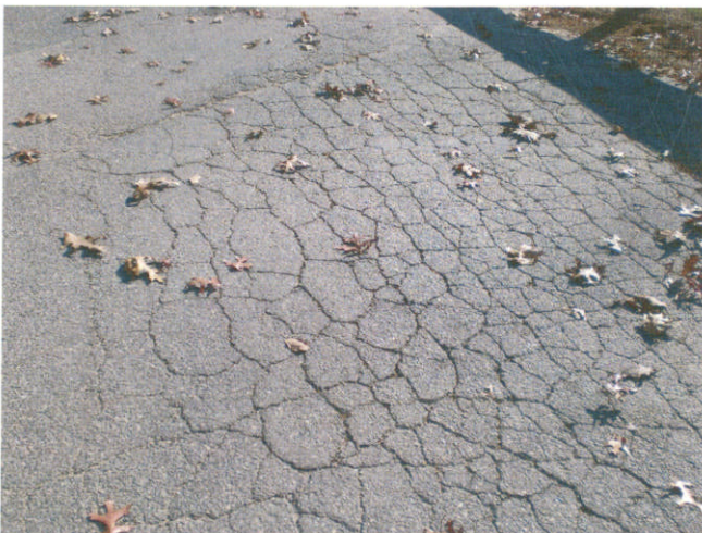
Cracks in pavement
