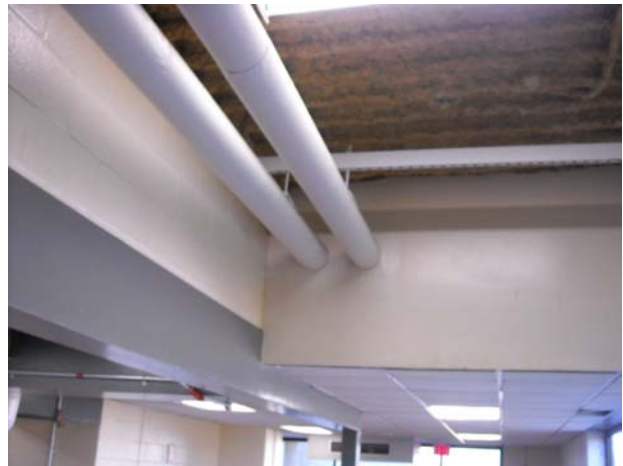
Typical Hot Water Piping in Corridors and Above Ceiling
