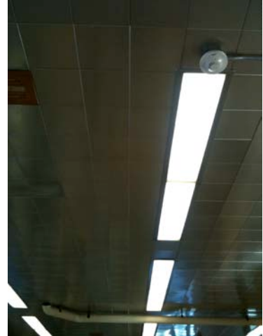
Typical Heat Detector
