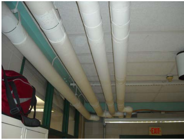
Typical Hot and Chilled Water Piping in Corridors
