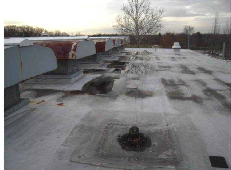
DETERIORATING ROOF TOP UNITS / MINIMAL ROOF DRAINS
