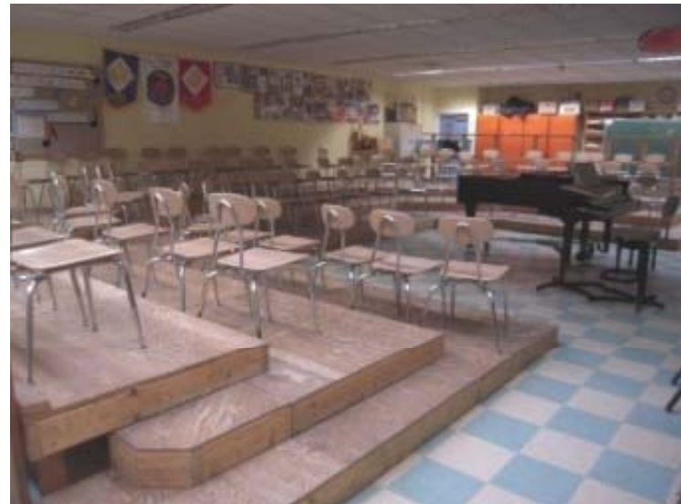
INACCESSIBLE PLYWOOD RISERS IN CHORAL ROOM
