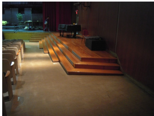
Inaccessible floor slope and stage
