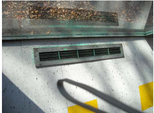
Cafeteria Floor Diffusers
