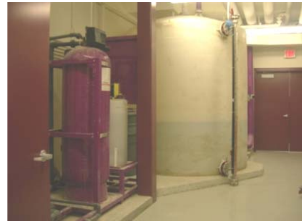
Rain Water Cistern
