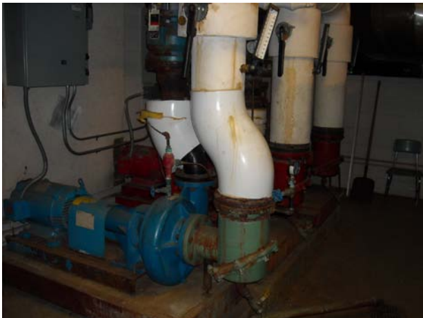
Hot Water Pumps in Boiler Room
