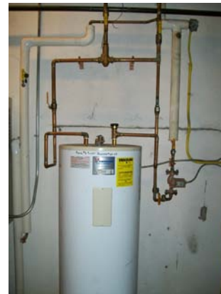
Building "H" electric wtr heater
