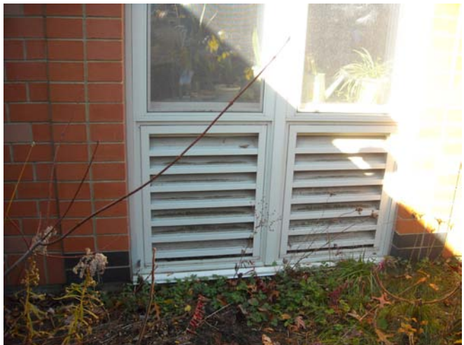
Typical Unit Ventilator Intake Louver
