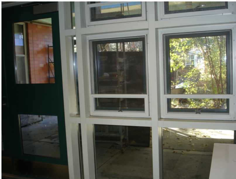
Figure 14. Typical modification to original curtain wall at courtyard exterior wall in Building S. These modifications were made in the 1990s.
