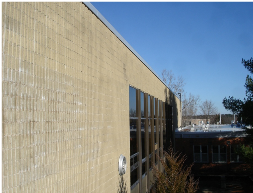
Figure 18. Condition of exterior wall at library.
