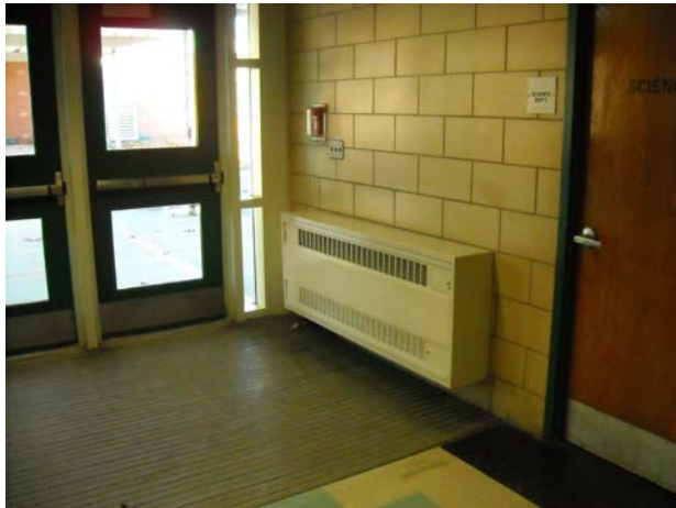
Typical Wall Type Cabinet Unit Heater
