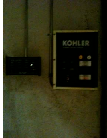
Remote Generator Annunciator
