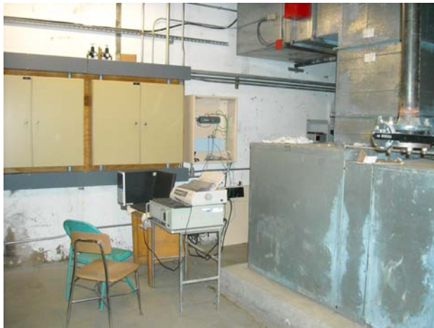
Front End Workstation – Building H Mechanical Room
