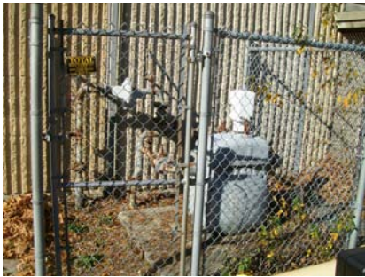
Building "I" gas meter
