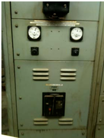
Main Circuit Breaker
