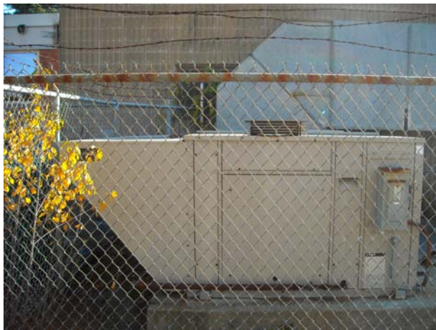
Packaged AC Unit - Building I
