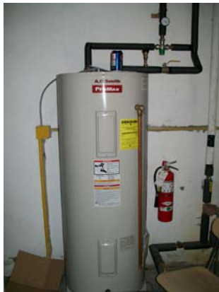
Building "A" electric wtr heater
