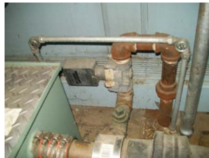
Kitchen automatic gas shutoff
