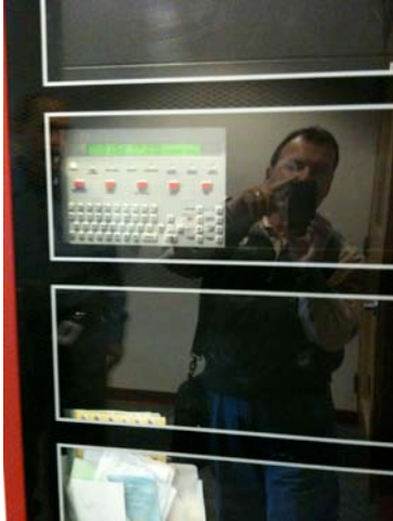
Main Fire Alarm Panel
