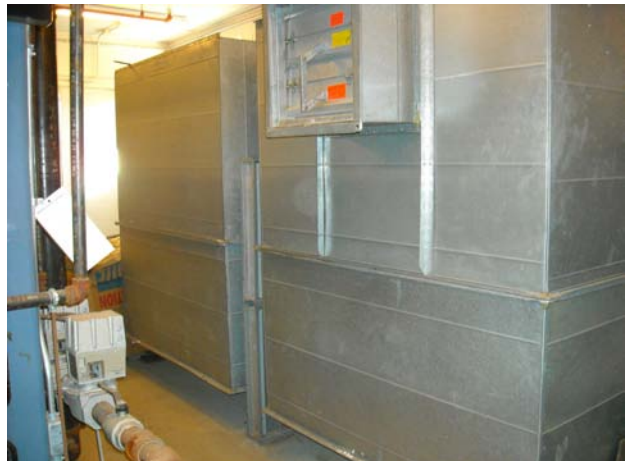
Boiler Room Combustion Air
