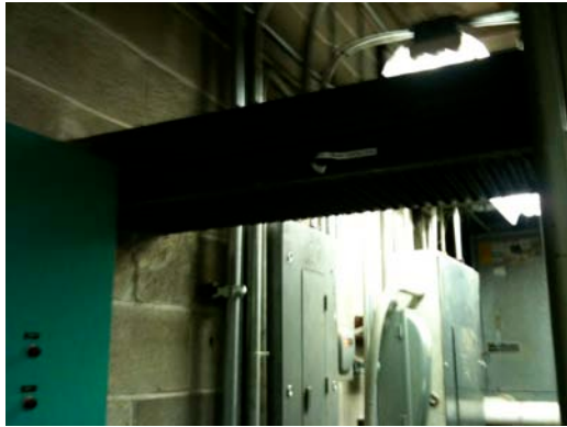
Typical panelboard with live bus exposed.
