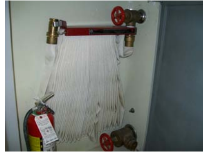
Fire Hose Cabinet
