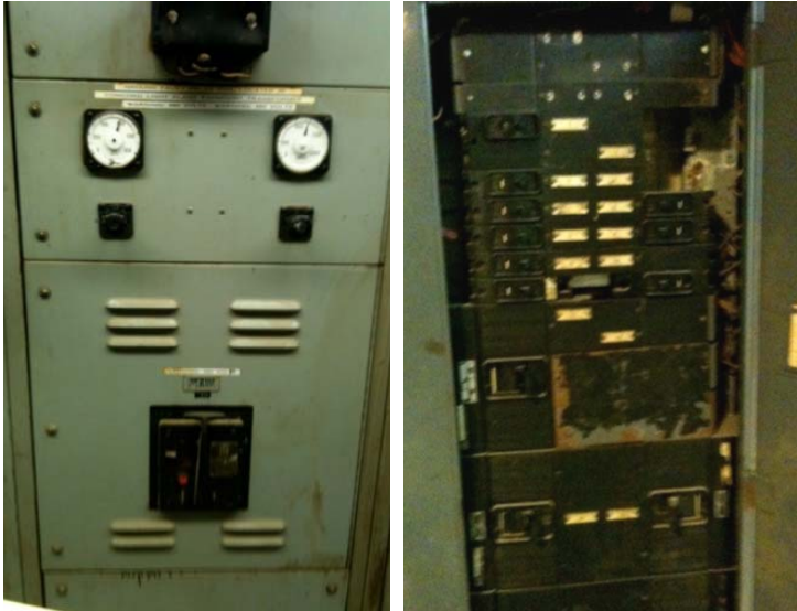
OUTDATED AND DETERIORATING ELECTRICAL PANELS
