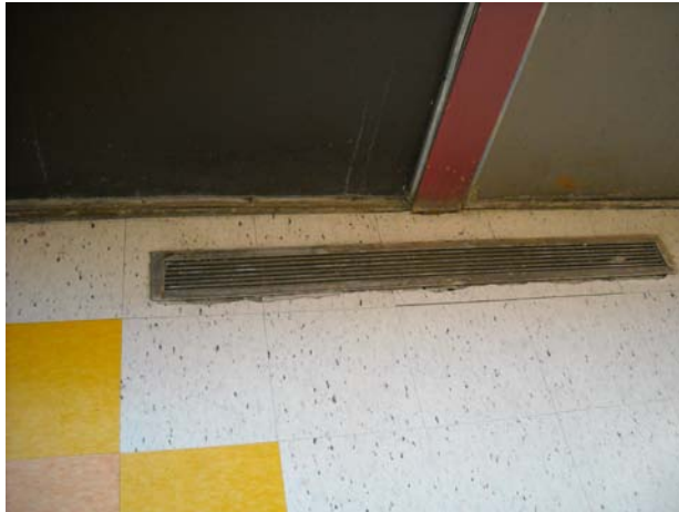
Cafeteria Floor Diffusers
