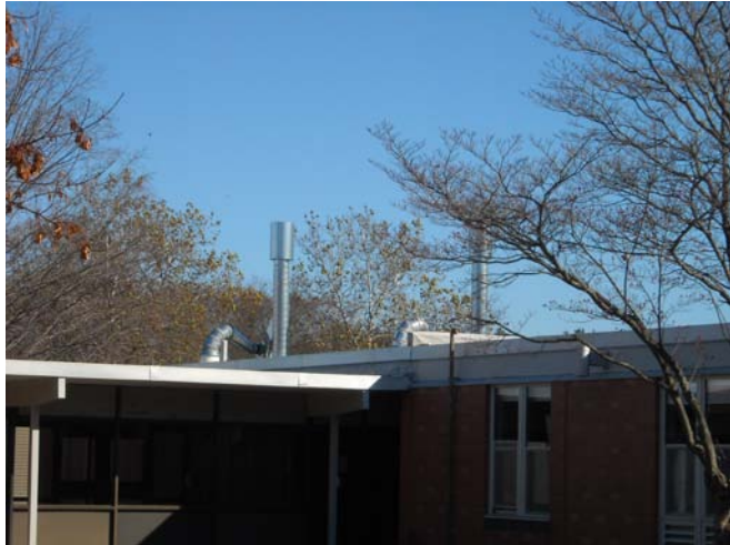
Building S – Fume Hood Exhaust Fans
