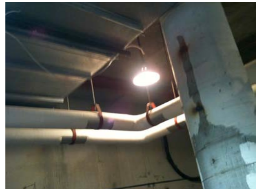
Mechanical Room Lighting
