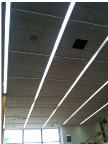
Library/Media Center Lighting
