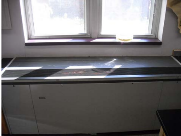
Typical Classroom Unit Ventilation
