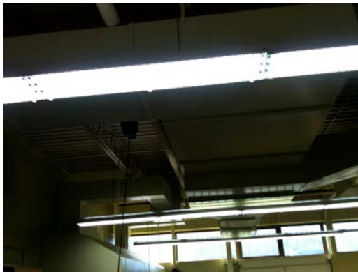
Typical Classroom Lighting
