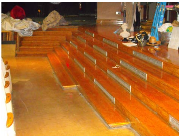
Auditorium Return Air Grilles
