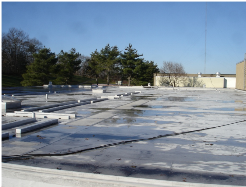
Figure 26. Overall view of ponding water at PVC roofs.
