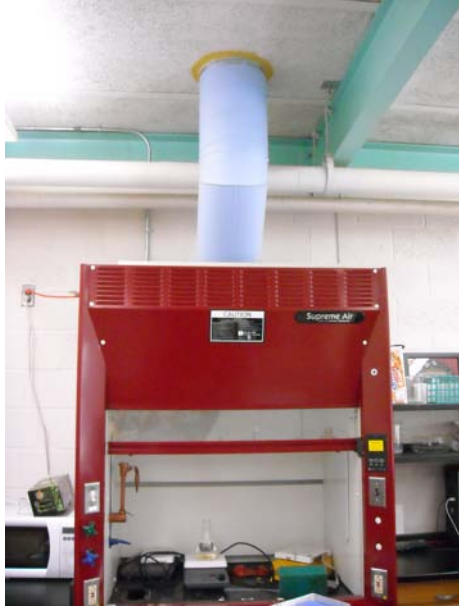
Building S – Fume Hoods
