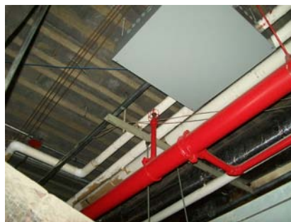
Mechanical Room upright sprinkler
