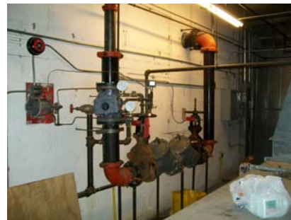
Building "H" sprinkler service
