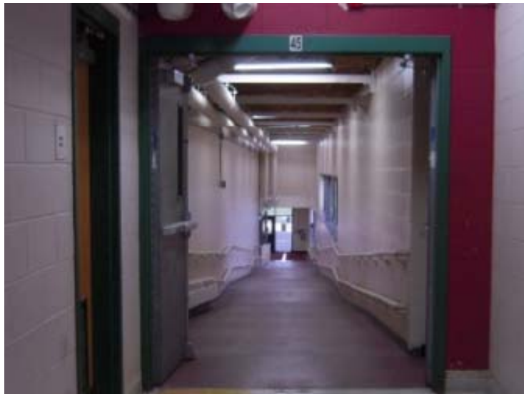
NONCOMPLIANT RAMP DOWN TO LOWER GYM
