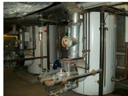
Lower Gym gas-fired water heaters
