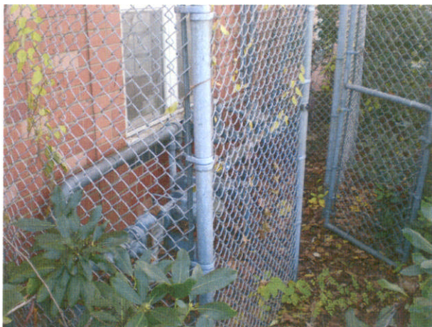
Gas regulator for school at Art Building
