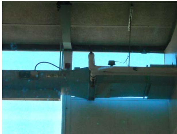
HV-7 Upper Gym Ceiling mounted H&V Unit
