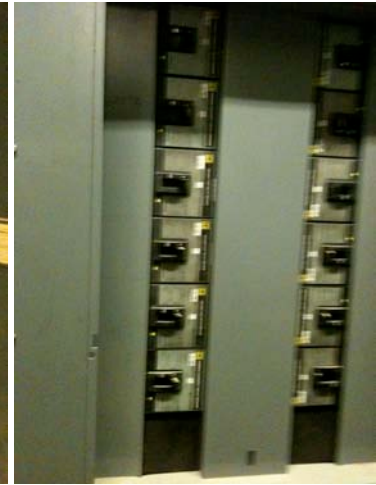
Typical Panel replaced in the 1990's
