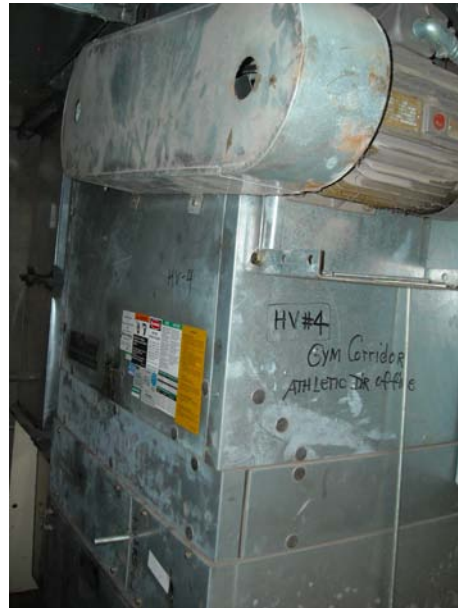
HV-4 Gym Office and Corridor H&V Unit
