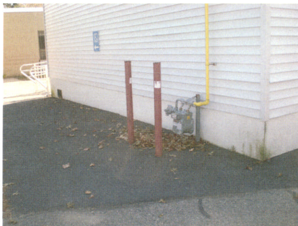
Gas meter at trailer
