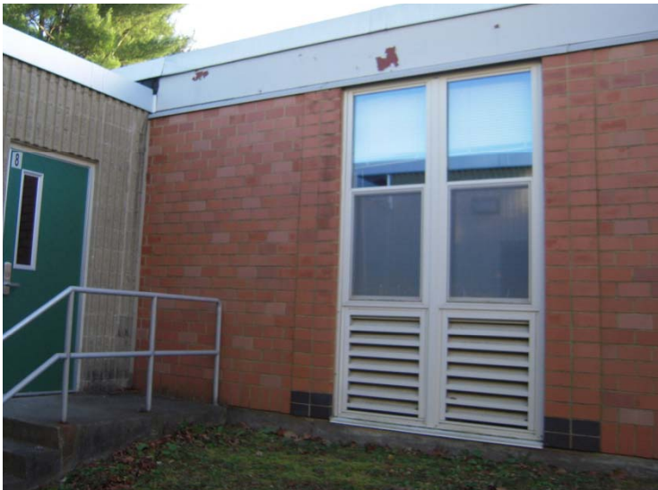
1990'S BUILDING ENVELOPE RENOVATION / LOUVERS TOO CLOSE TO GROUND
