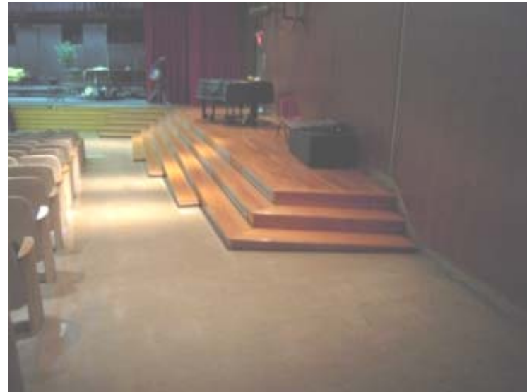
INACCESSIBLE AUDITORIUM STAGE AND NONCOMPLIANT SLOPED FLOOR
