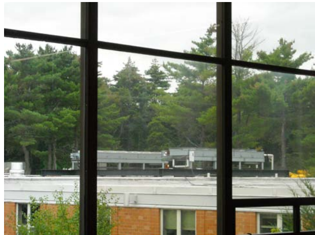
Air Cooled Condensing Units on Building H Roof
