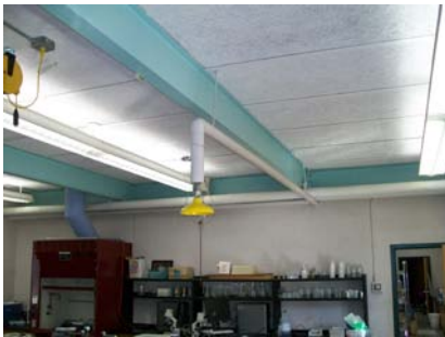
Classroom emergency shower
