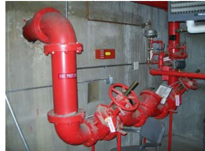
Lower Gym sprinkler service
