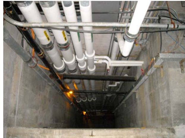
Hot and Chilled Water Piping in Tunnel
