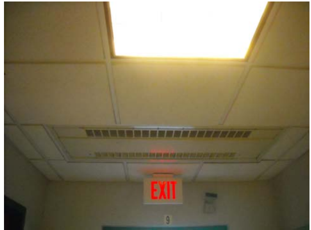
Type Ceiling Mounted Cabinet Unit Heater
