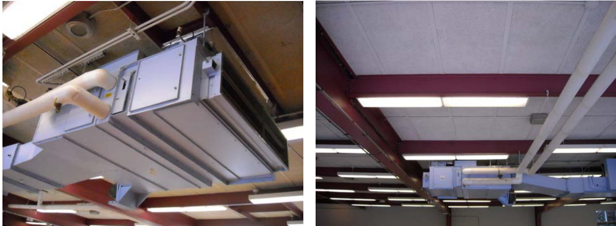
Cafeteria HV-8A & 8B Heating and Ventilation Units
