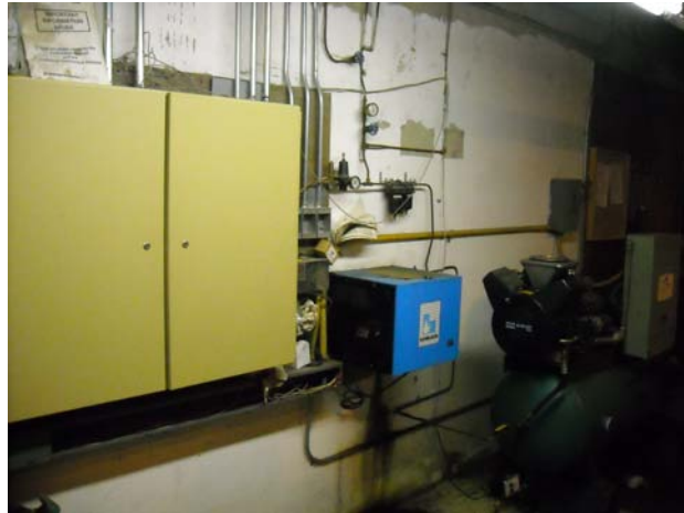
Typical ATC Control Panel
