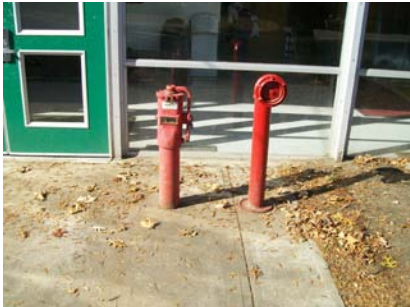
Lower Gym PIV & Fire Department connection
