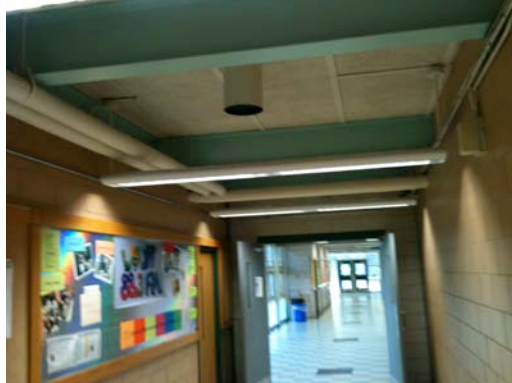
Typical Corridor Lighting
