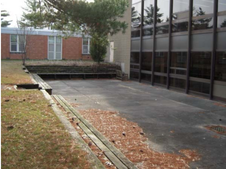
DETERIORATING SITE ELEMENTS
