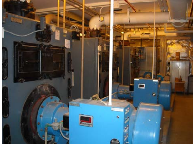
Boiler Plant – Building H
