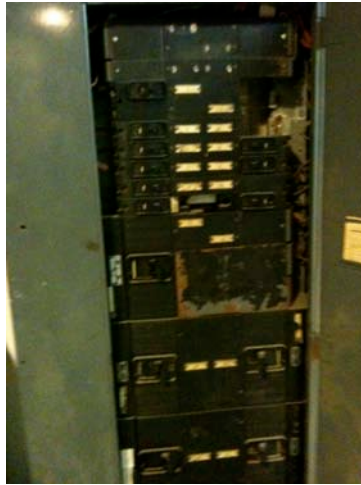
Typical Original Distribution Panel
