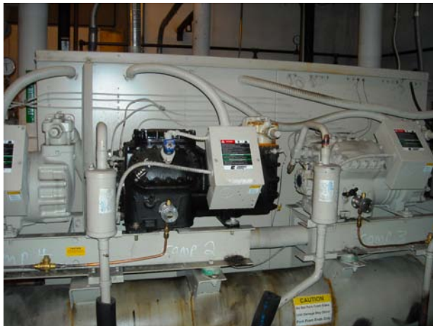
Chiller in Building H Basement Mechanical Room
