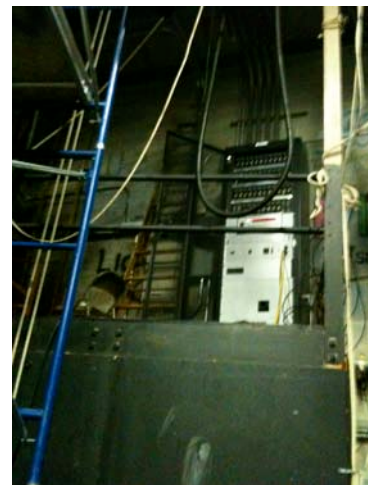
Auditorium House Dimming System
