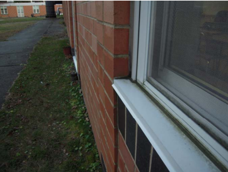
NEWER WINDOWS HAVE SILLS PITCHING BACK TO BUILDING
