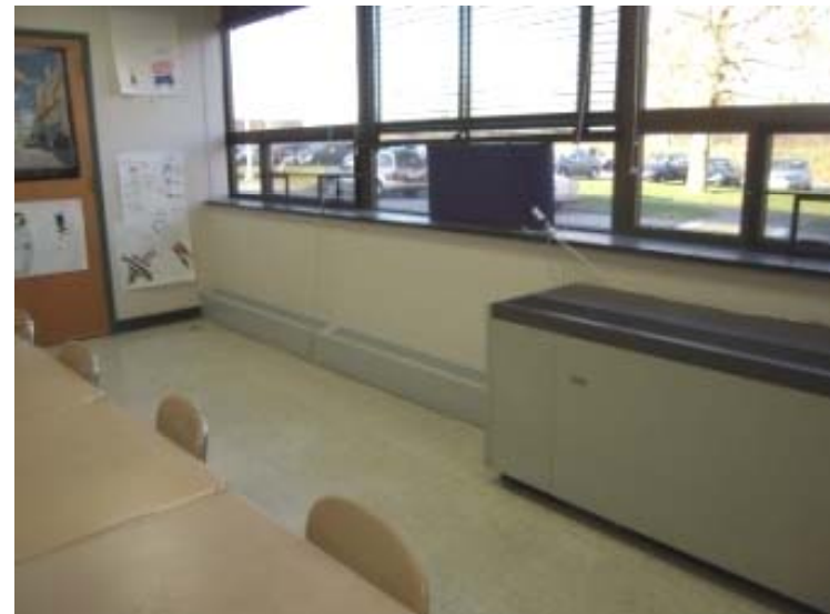
UNIT VENTILATORS IN CLASSROOMS ARE NOISY, INEFFICIENT AND HARD TO MAINTAIN
