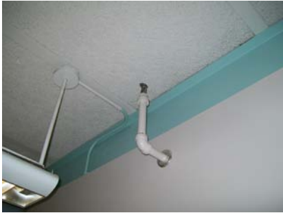
Building "H" Corridor sprinkler
