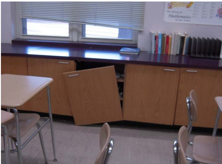
90'S CASEWORK: BROKEN HINGES ON MANY CABINET UNITS
