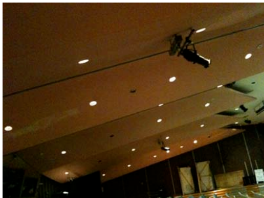
Auditorium Housing Lighting
