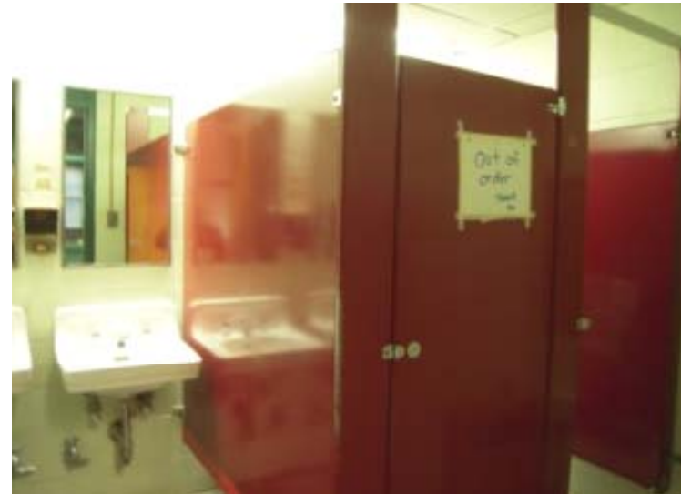
HIGH MAINTENANCE AND INEFFICIENT PLUMBING / INACCESSIBLE TOILET ROOMS
