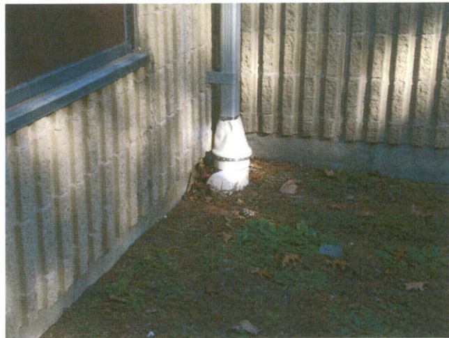
Down spout between S and L-Buildings
