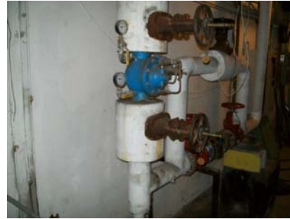
Water meter and PRV
