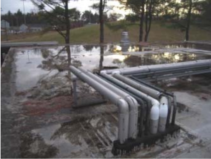
PONDING ON ROOF / EXPOSED PIPING
