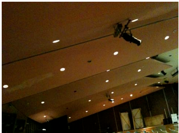
Auditorium Supply Air Diffusers
