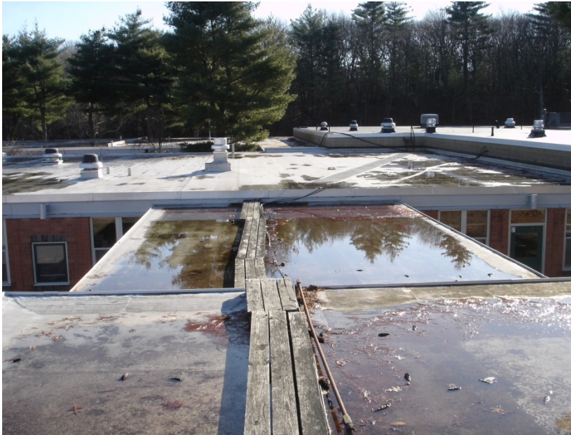
Figure 27. Severe ponding water at roof membranes between buildings H and S at PVC roofs.
