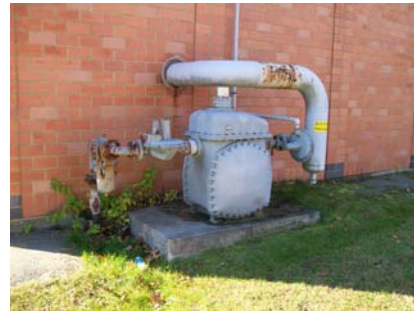
Building "H" gas meter
