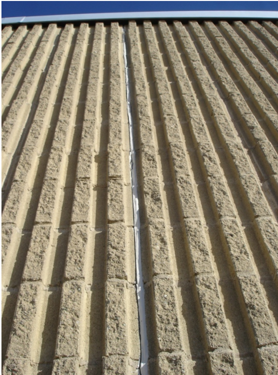
Figure 21. Typical condition of sealant joints at 1970s construction.
