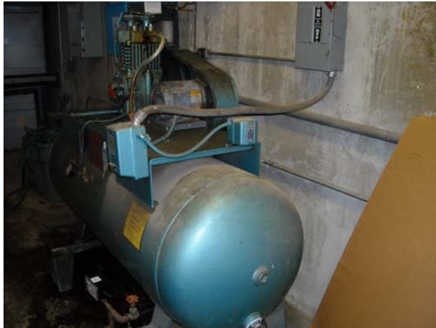
ATC System Compressor – Gym Mechanical Room
