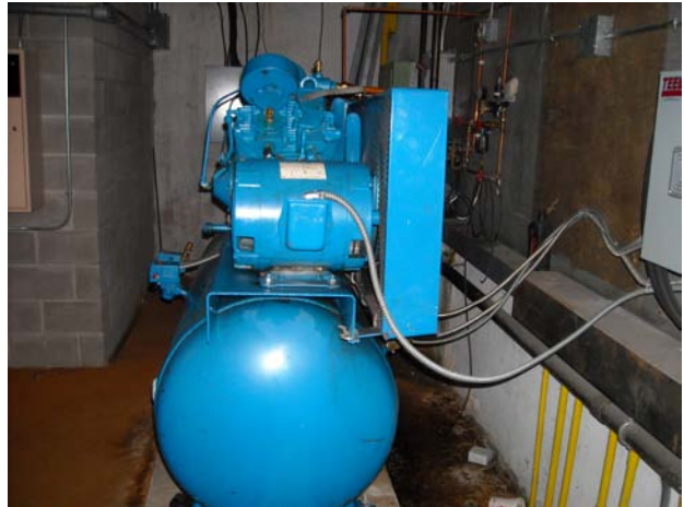
ATC System Compressor Building H Basement Mechanical Room
