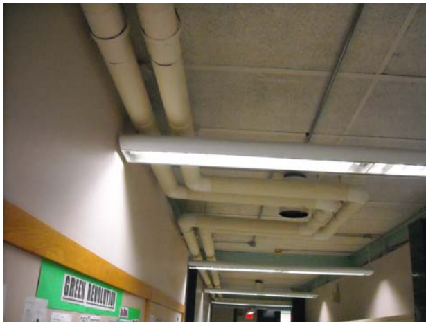
Hot Water Piping with Expansion Loop in Corridor
