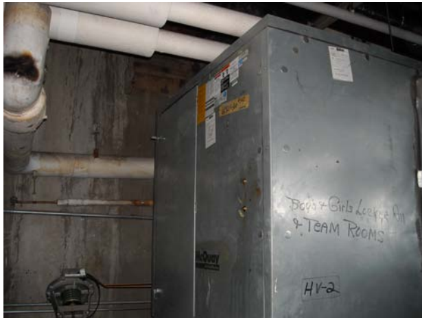
HV-2 Boys & Girls Locker Room H&V Unit
