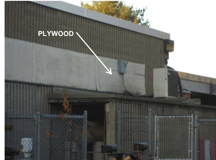
DELAMINATING PLYWOOD PANELS
