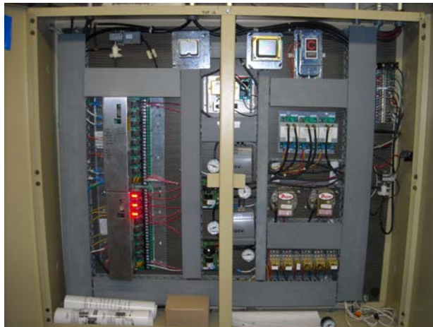
Typical ATC Control Panel
