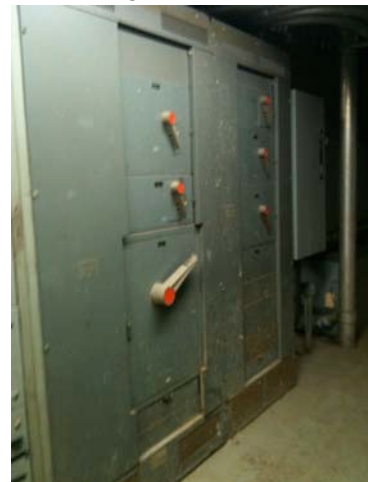
1973 Modification to Main Switchboard
