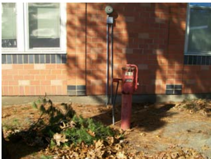
Building "H" PIV
