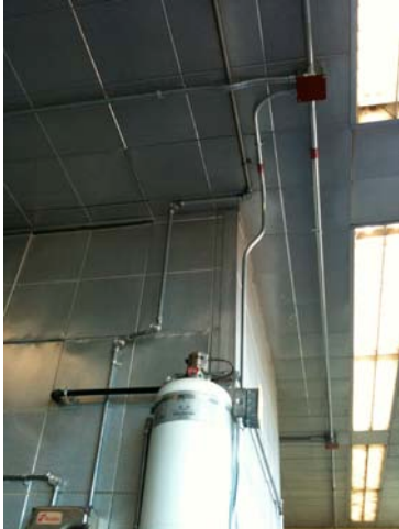
Hood Suppression System
