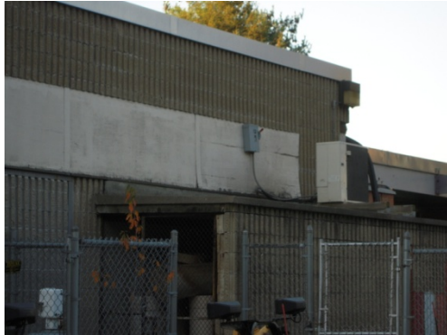
Ribbed block/delaminating plywood panels
