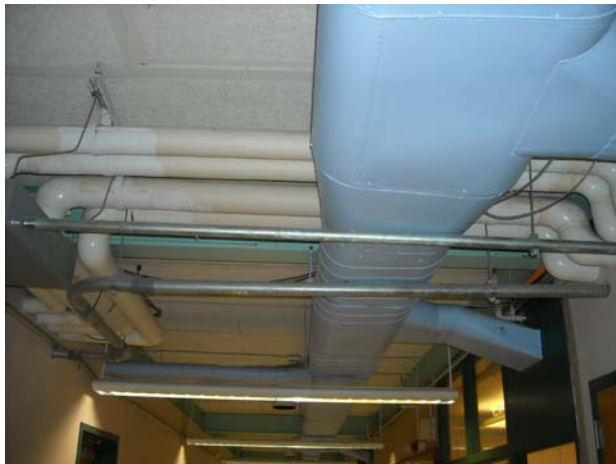
Typical General Exhaust Ductwork Serving Classrooms
