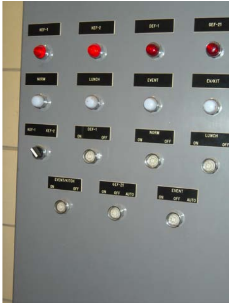
Typical Equipment Status Indicator Panel
