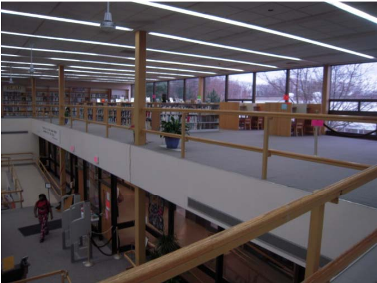
NONCOMPLIANT GUARDRAILS IN LIBRARY
