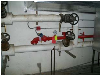
Building "A" Basement Mech. Room control valve & flow switch
