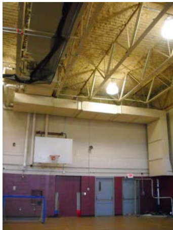
HV-6B - Lower Gym Heating & Ventilation System (similar to HV-6A)
