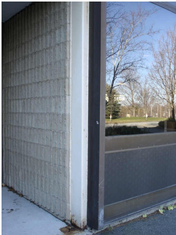
Figure 20. Masonry/curtain wall interface with steel structure penetrating the building enclosure at the library/cafeteria.
