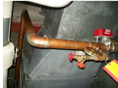
Building "I" Basement Mech. Room control valve & flow switch
