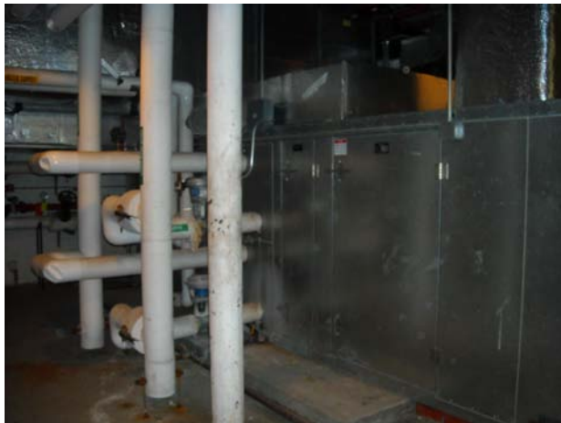
HVAC-3 – Auditorium Air Handling Unit
