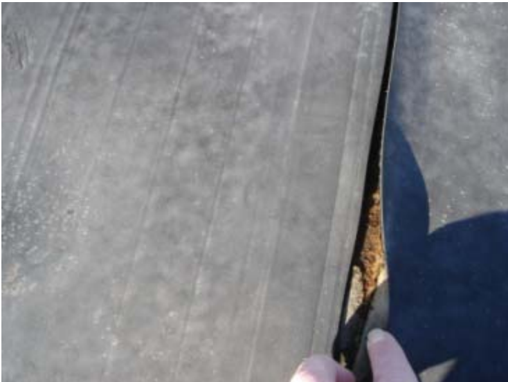
OPEN SEAMS IN EPDM ROOFING
