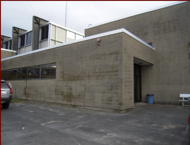
POORLY INSULATED MASONRY WALLS WITH WEAK AIR BARRIER SYSTEM
