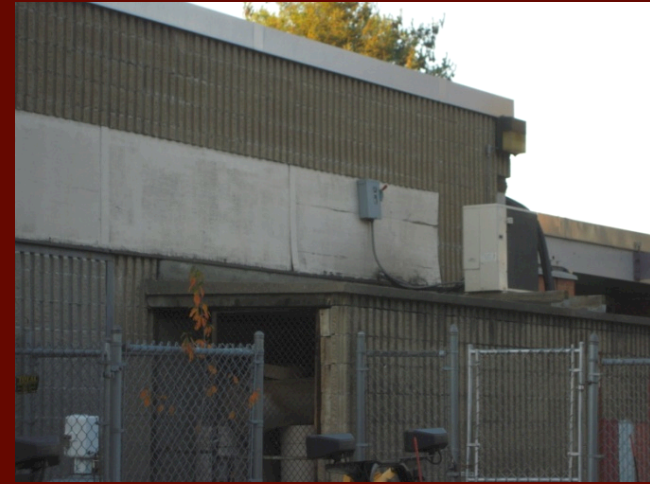
DELAMINATING PLYWOOD PANELS
