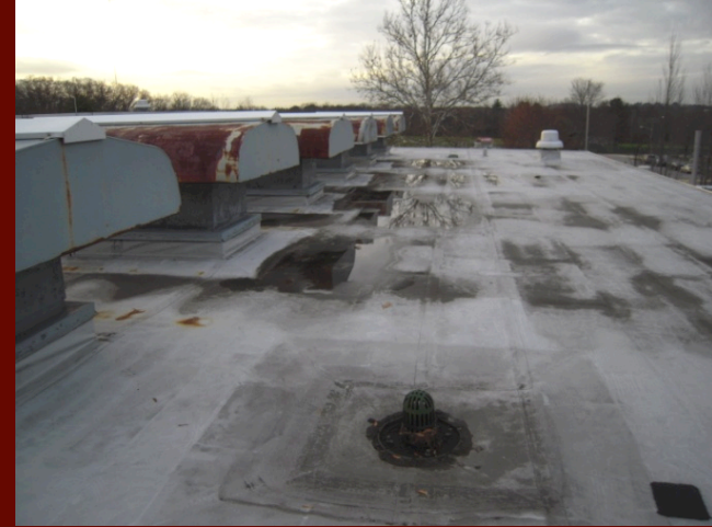
DETERIORATING ROOF TOP UNITS / MINIMAL ROOF DRAINS
