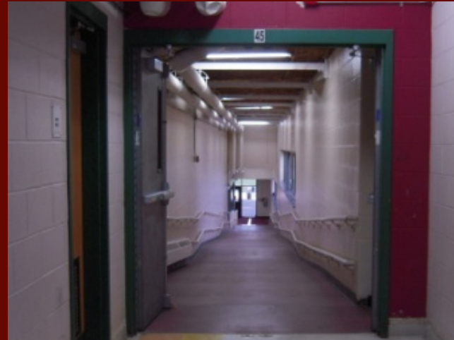
NONCOMPLIANT, INACCESSIBLE AREAS
