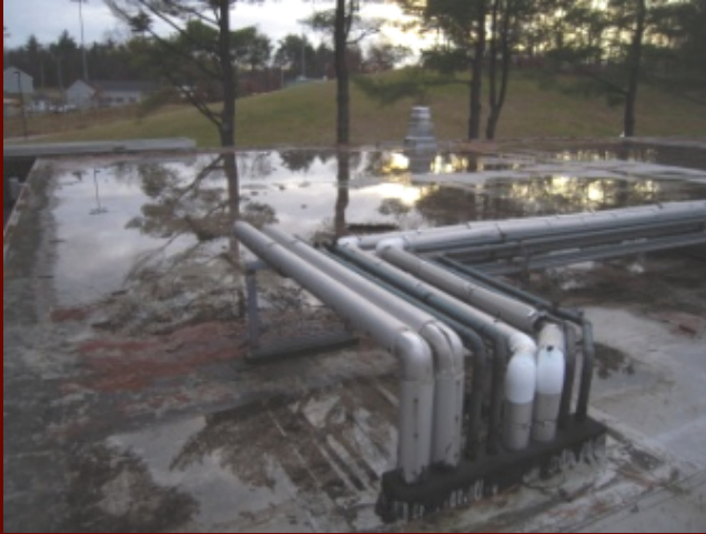
PONDING ON ROOF / EXPOSED PIPING
