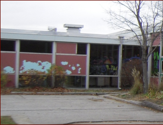
1960's NONINSULATED STOREFRONT SYSTEM WITH PEELING PAINT ON METAL PANELS
