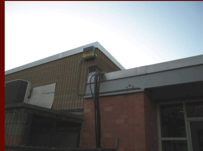
EXPOSED UTILITY LINES
