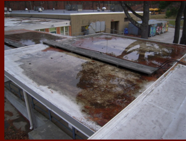
PONDING ON ROOF / DETERIORATING WOOD PLANK WALKING PADS
