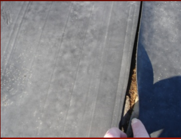
OPEN SEAMS IN EPDM ROOFING
