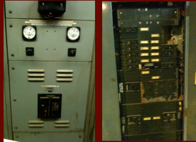
OUTDATED AND DETERIORATING ELECTRICAL PANELS
