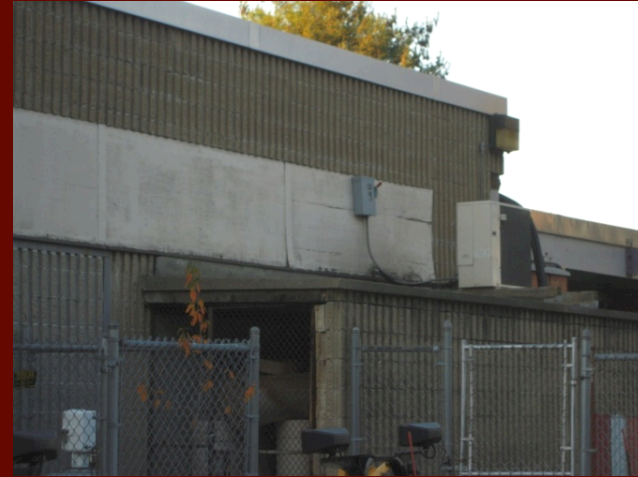
DELAMINATING PLYWOOD PANELS
