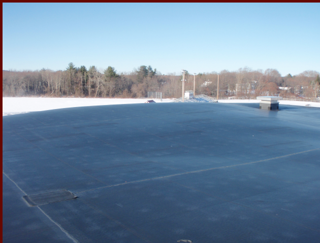
OPEN SEAMS IN ROOFING
