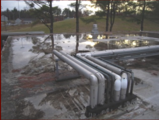
PONDING ON ROOF / EXPOSED PIPING
