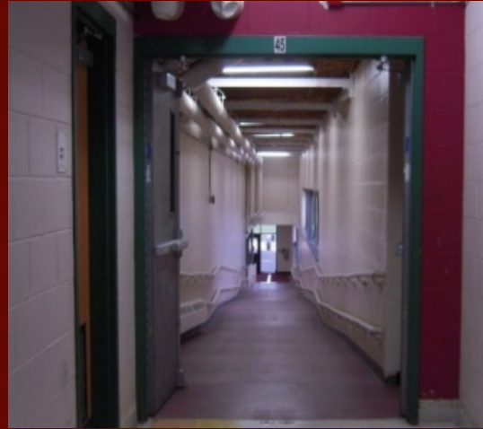
NONCOMPLIANT, INACCESSIBLE AREAS
