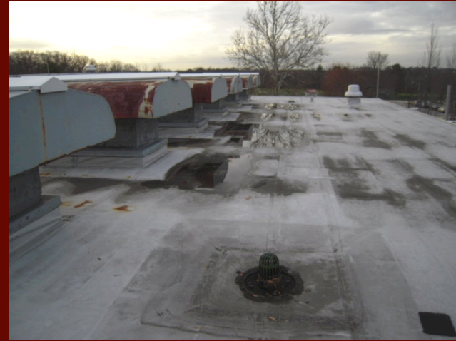
DETERIORATING ROOF TOP UNITS / MINIMAL ROOF DRAINS
