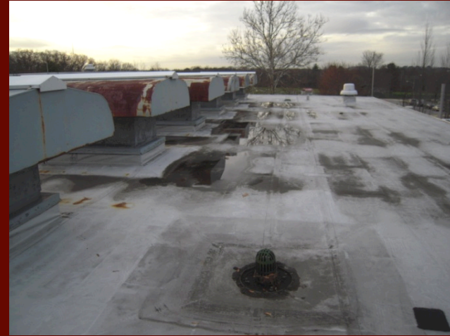
DETERIORATING ROOF TOP UNITS / MINIMAL ROOF DRAINS
