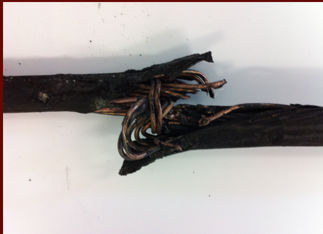
CABLE FROM RECENT ELECTRICAL FAILURE
