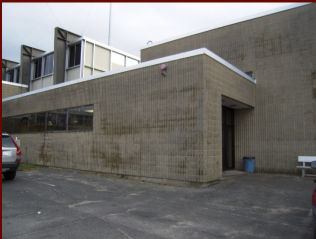
POORLY INSULATED MASONRY WALLS WITH WEAK AIR BARRIER SYSTEM
