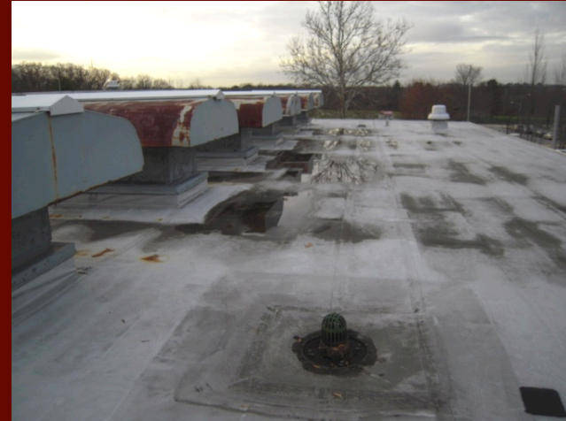
DETERIORATING ROOF TOP UNITS / MINIMAL ROOF DRAINS
