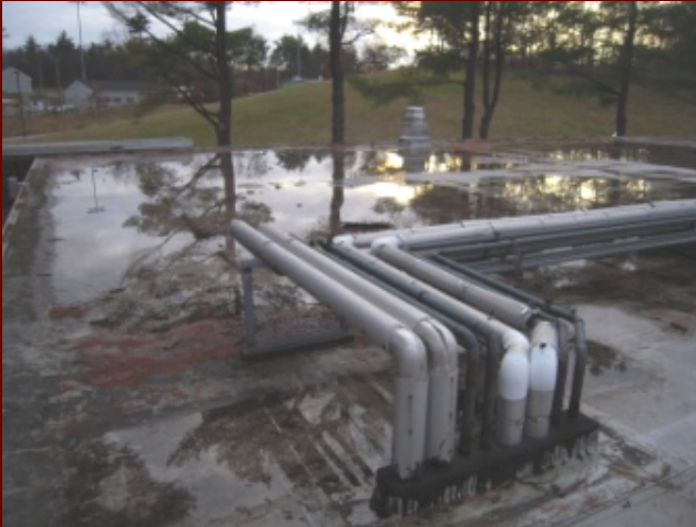
PONDING ON ROOF / EXPOSED PIPING
