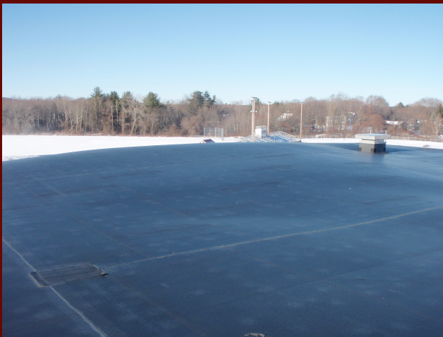
OPEN SEAMS IN ROOFING
