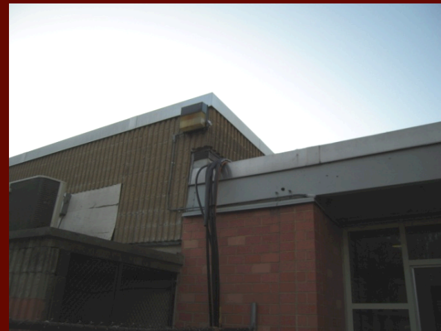
EXPOSED UTILITY LINES
