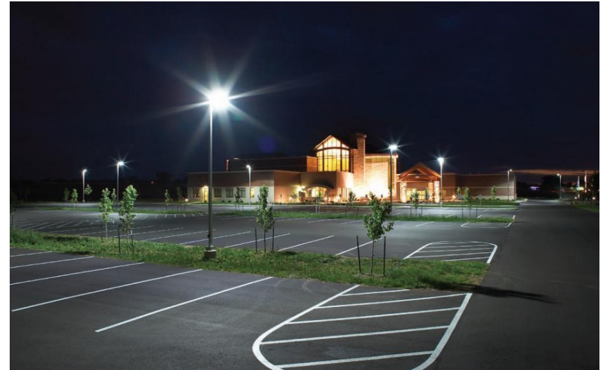
LED Site Lighting
