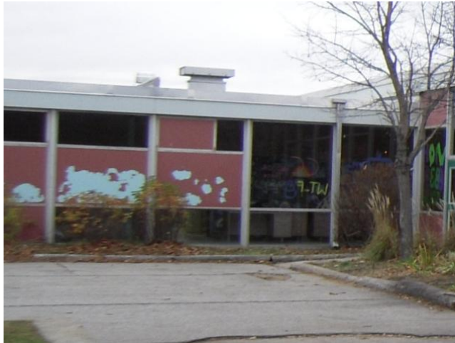
1960's NONINSULATED STOREFRONT SYSTEM WITH PEELING PAINT ON METAL PANELS
