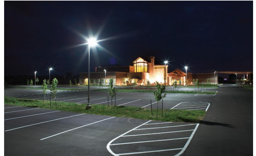
LED Site Lighting
