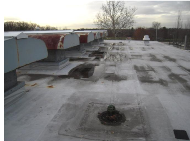
DETERIORATING ROOF TOP UNITS / MINIMAL ROOF DRAINS
