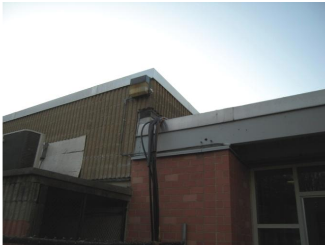
EXPOSED UTILITY LINES
