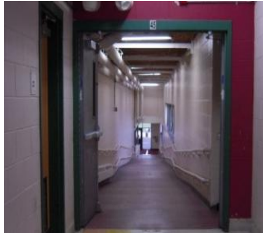
NONCOMPLIANT, INACCESSIBLE AREAS
