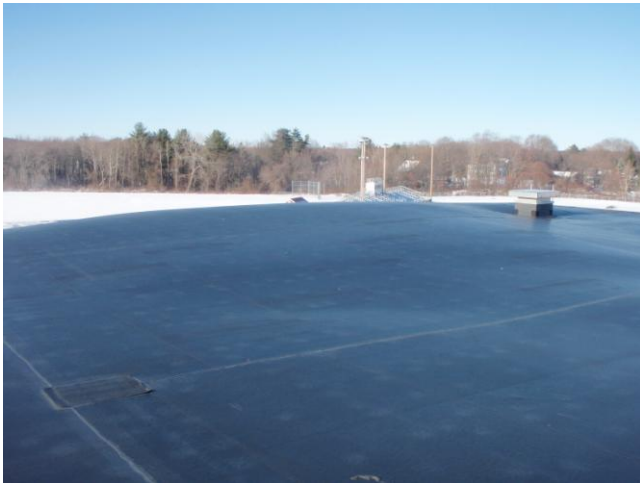
OPEN SEAMS IN ROOFING
