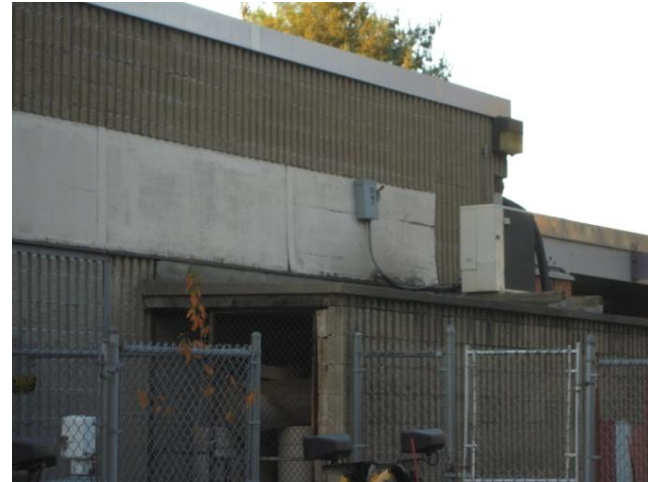
DELAMINATING PLYWOOD PANELS
