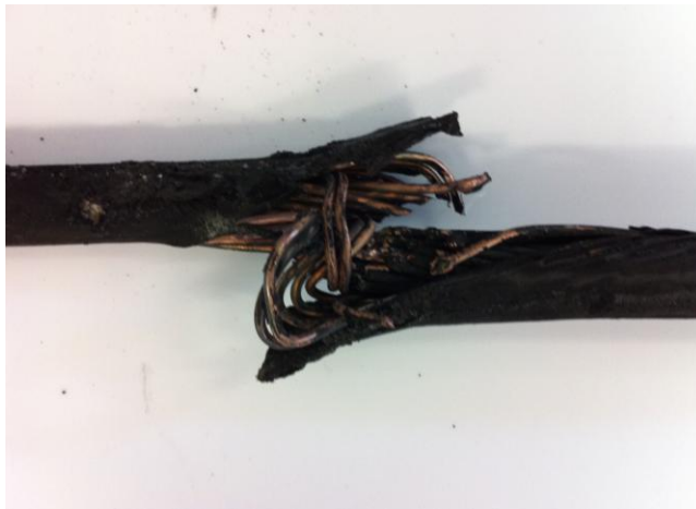
CABLE FROM RECENT ELECTRICAL FAILURE
