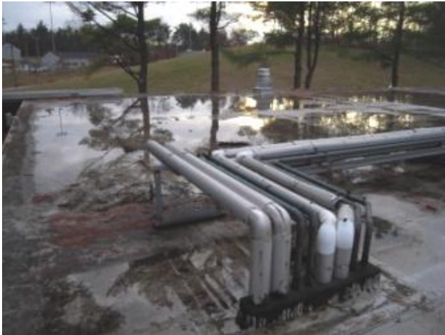
PONDING ON ROOF / EXPOSED PIPING
