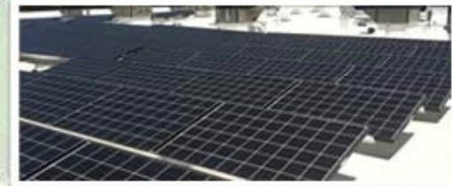
Solar Power Generation
